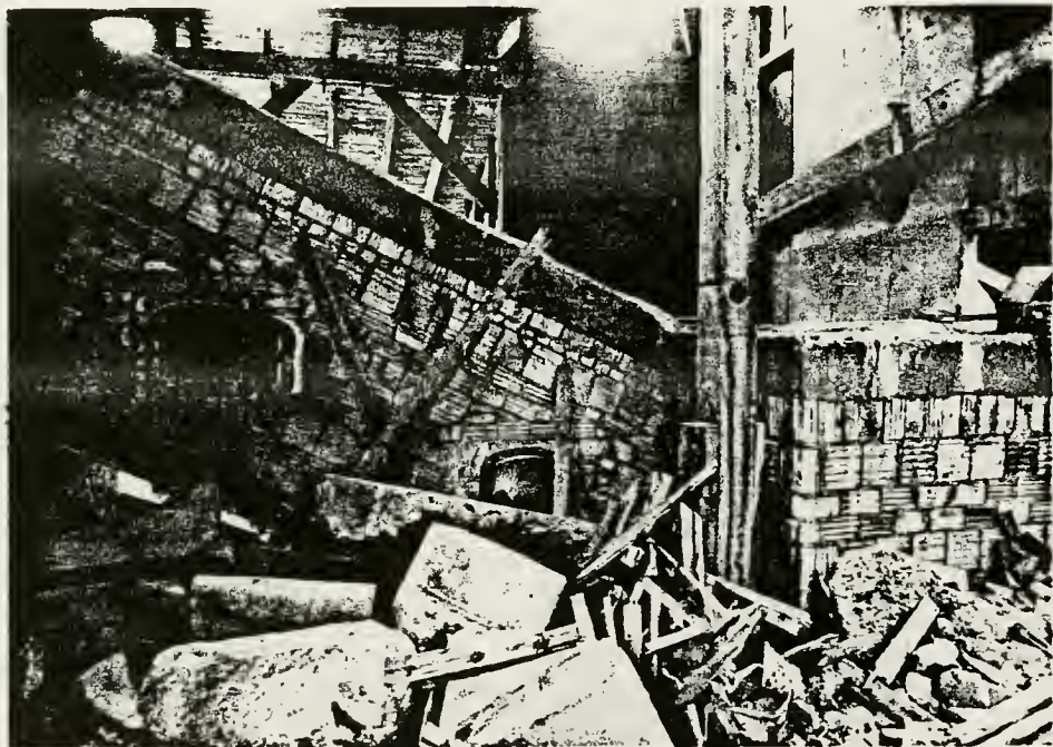
Figure 161. Arsenic plant (structure #59) showing detail of the flue entering the primary kitchen, west view.
